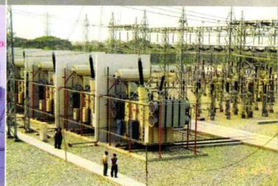
Khulna (south) substation constructed under NDF finance
