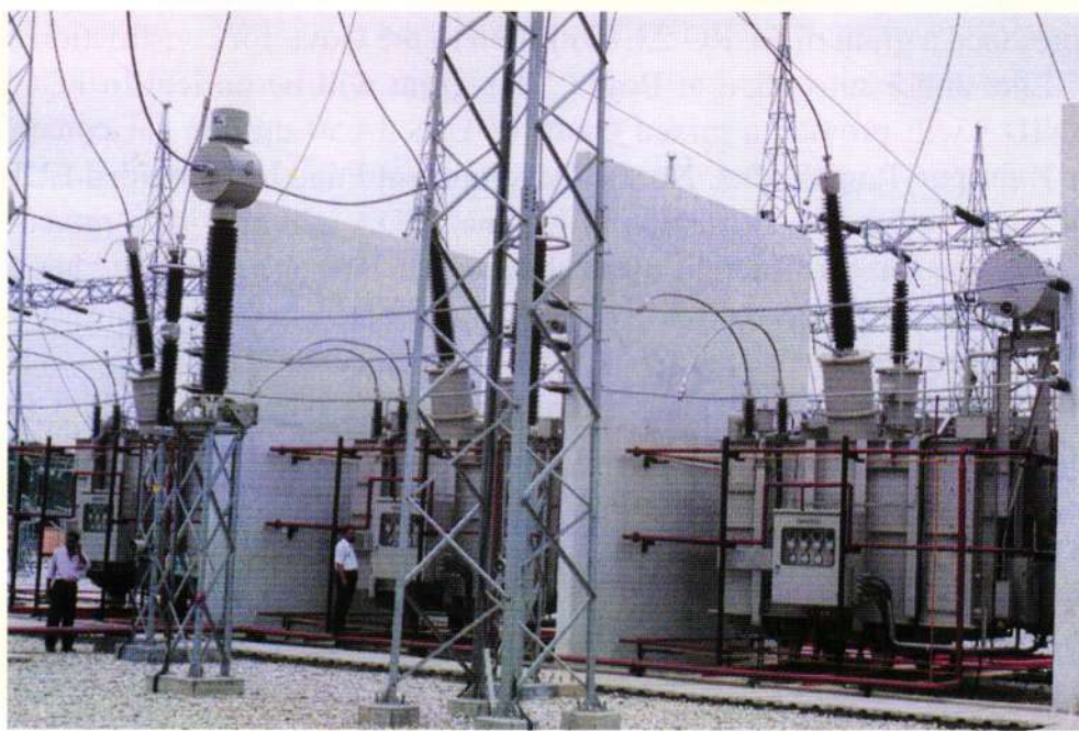
Transformers at Barapukuria 230/132 kV Sub-station
