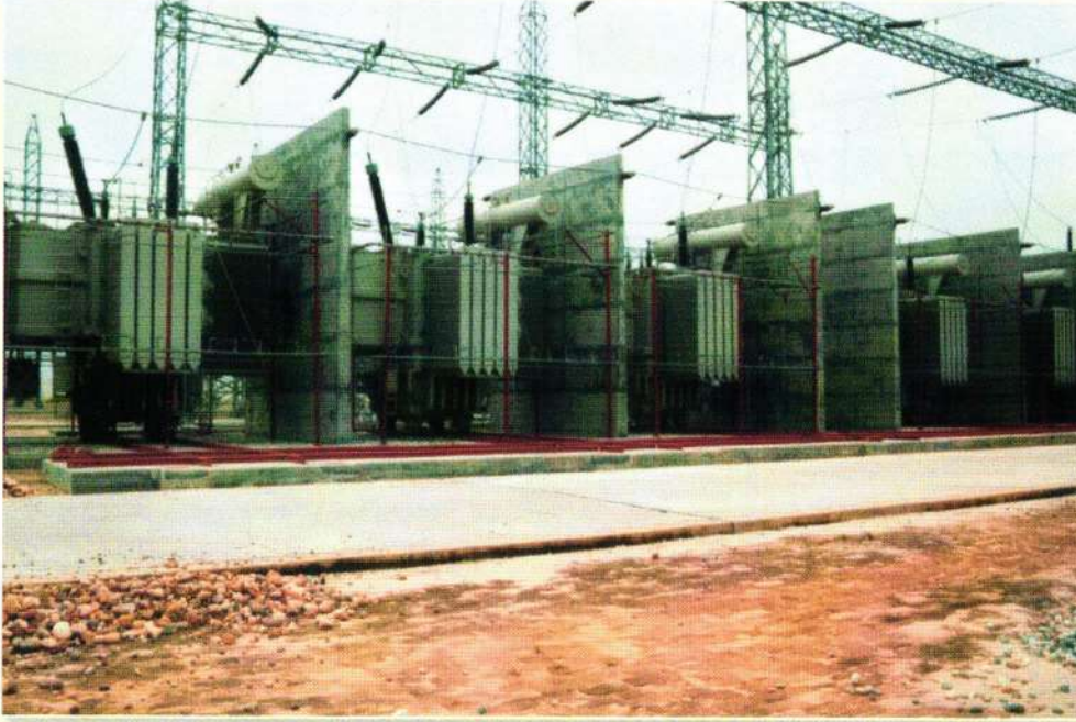
Transformers at Aminbazar 230/132 kV Sub-station
