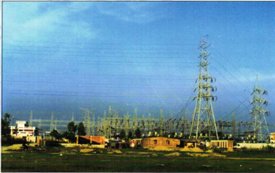
Ullon-Bashundhara 132 kV Turn-in-line to Rampura Substation on Four-Circuit Tower
