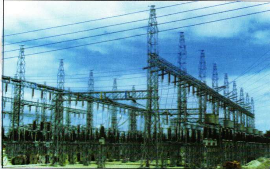
A section of Rampura 230/132kV Substation
