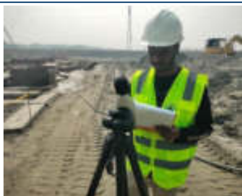
NL41 Near 132/33 kV GIS substation at Phultola
