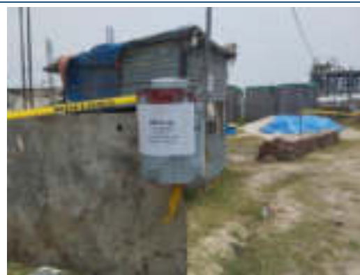
Phultola Substation (Package 7)
