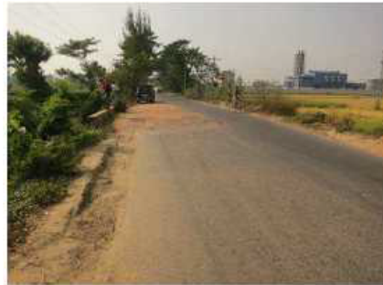
Cracks and other asphalt damage are seen at various locations along the road.
