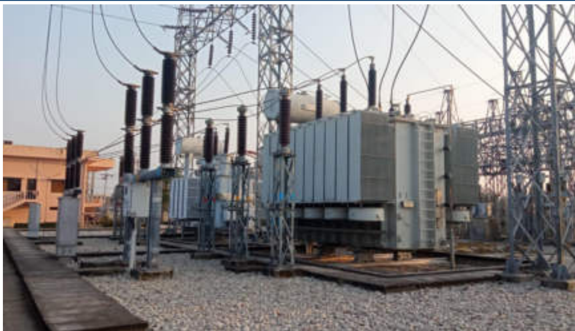
Switchyard of Existing Satkhira Substation
