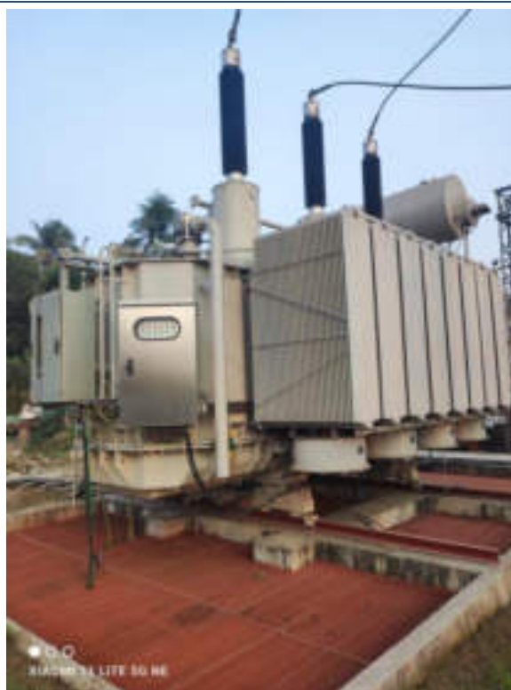
Switchyard of Existing Kushtia Substation
