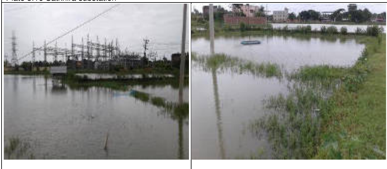
Plate 3.17 Satkhira substation and the adjacent land (3 acre) identified for the bay extension
